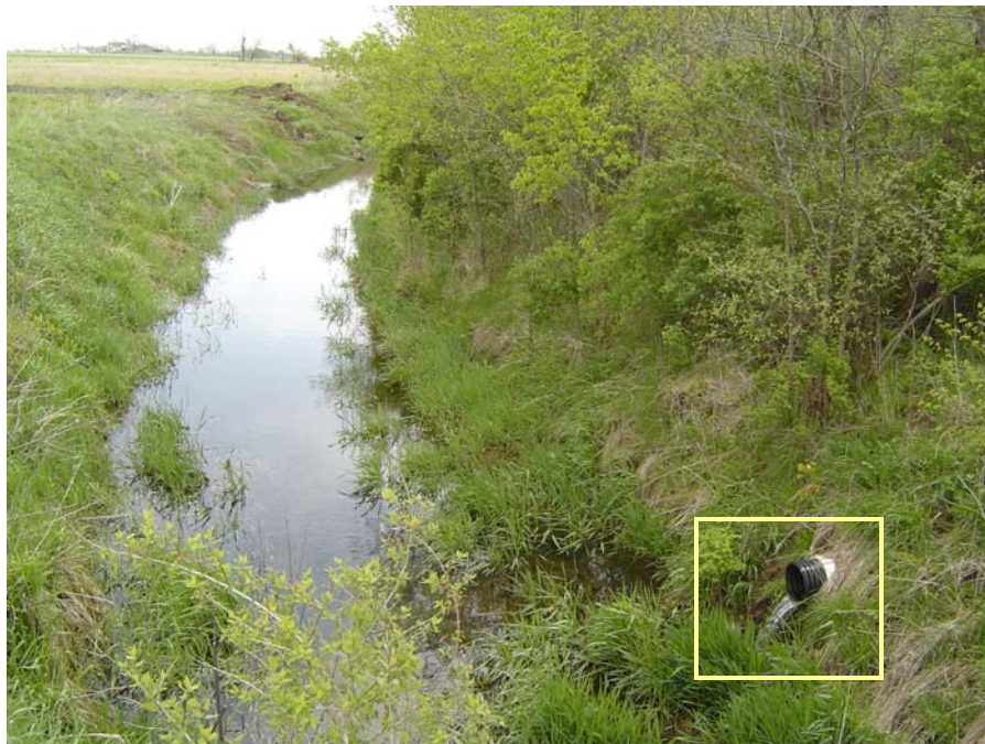
Mounts Run – Pipe discharging into stream.
